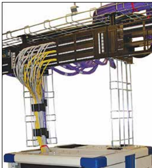
Out of Rack Connectivity Solution located above Active Cabinet
