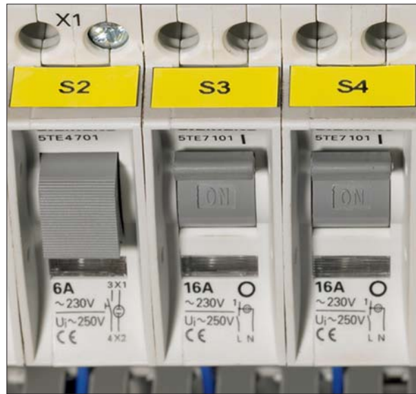
Clearly identified labels ensure easy network wire and cable management.
