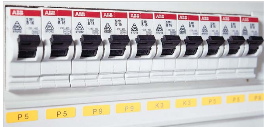
Helatag 860 switchgear application.
